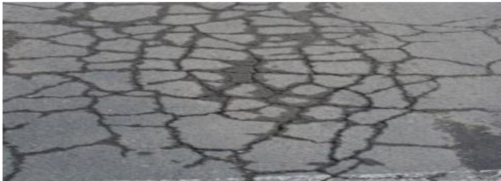
Fig.1: Alligator Cracks Formed in Flexible Pavements
