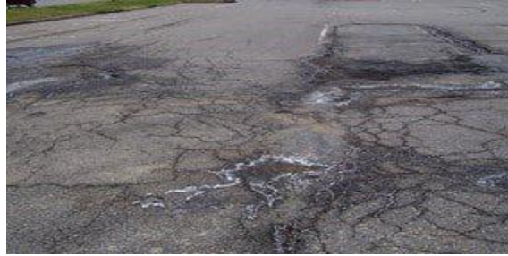
Fig 8: Effect of Rain on Pavement Design
