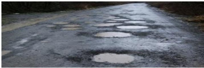
Fig.5: Potholes in Pavement
