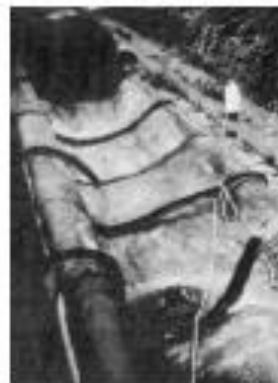
Pipe damage in
