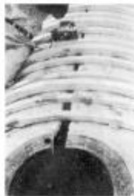
Burst pipe in power
